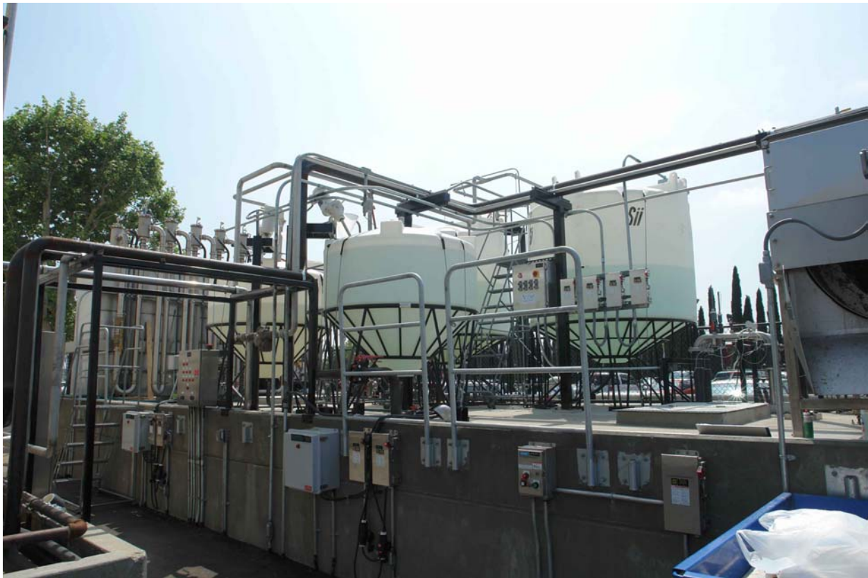
Figure 5. Actual photo of the system installed at PPI/Heinz plant at Chatsworth, California.
